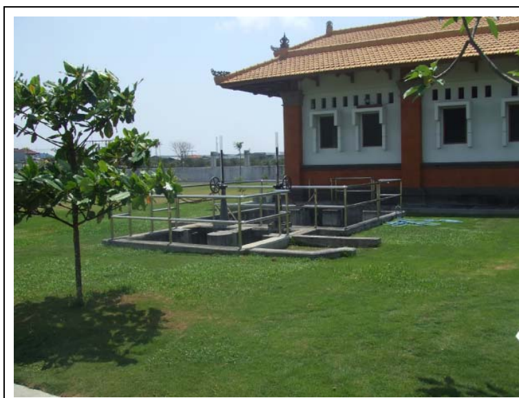
Picture 5.3.2 Pengolahan WWTP
