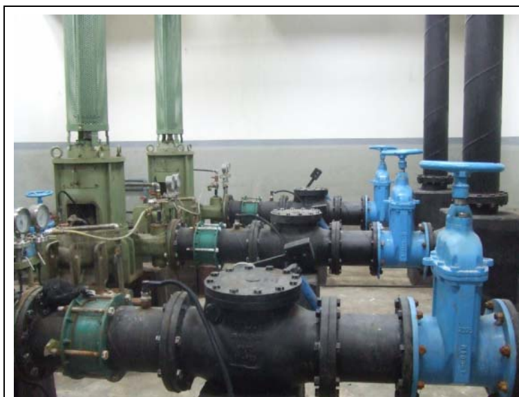
Picture 5.3.10 Sewerage Transmission Pumping Station
