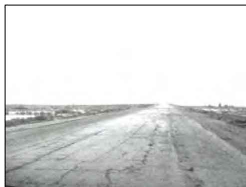
Surface has been damaged (near Tejen)
