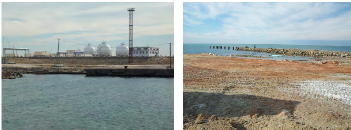
Figure 2.1.41 LPG Terminal (left) and Fishing Jetty (right, under construction) in Kiyarly Port
