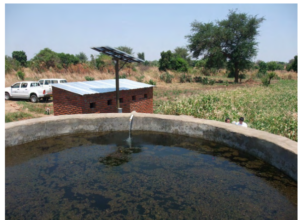
Photo 12 Site visit for PV irrigation system
