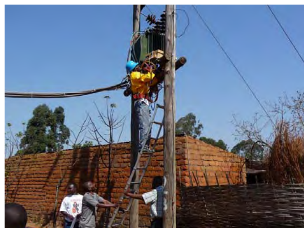
Photo 4 Final connection of data logger to the transformer
