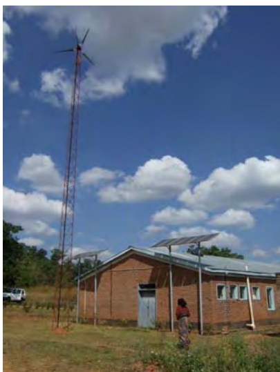
Photo 4: A wind and PV hybrid system (Main energy source is from PV because of no wind)
