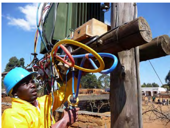
Photo 3 Checking connection of the transformer
