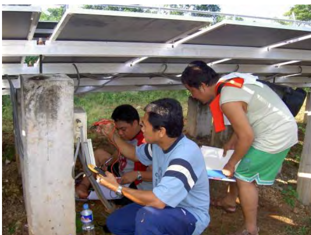
Check of PV array output
