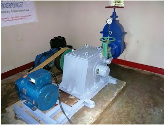
Turbine and Generator
