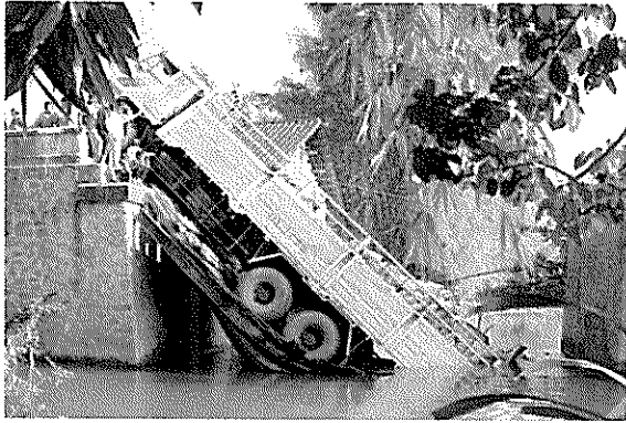
A bridge collapsed due to overloaded vehicle
