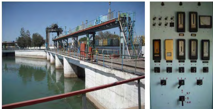
Figure 2-15 Intake Facility in the Dustlic Canal (Left) and Electric Control Panel for Intake Facility Operation (Right), photos taken in Sep. 2008.
