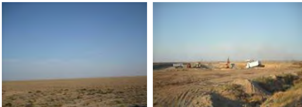
Figure 2-14 Koksarai regulating reservoir project site (left) / Canal construction site (right), photos taken in Sep. 2008. – Koksarai regulating reservoir is planned to be connected to the Syrdarya River by two canals. It is intended to alleviate flood damage during the winter season (stored water in the regulating reservoir) and to ensure water use during the irrigation period (released from the regulating reservoir to the river that is to be sent for farming). Prior to the construction of the regulating reservoir, canal excavation work had started.
