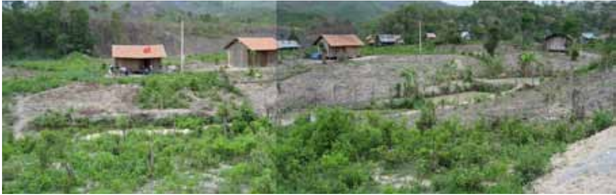
5 new ponds were made in line over the stream: most of earth works were finished (April 2008)
