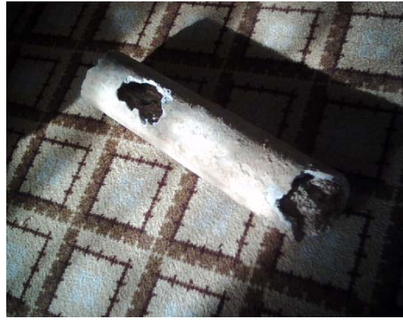
Damaged Asbestos Cement Pipe by penetration of Wooden Root
