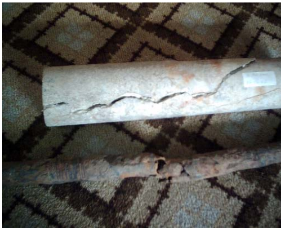
Cracked Asbestos Cement Pipe (above) and Corroded Steel Pipe (below)
