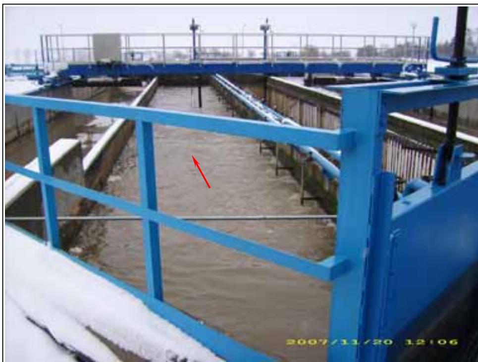
Pic.10 - Shumen WWTP: Detailed view of aeration tank
