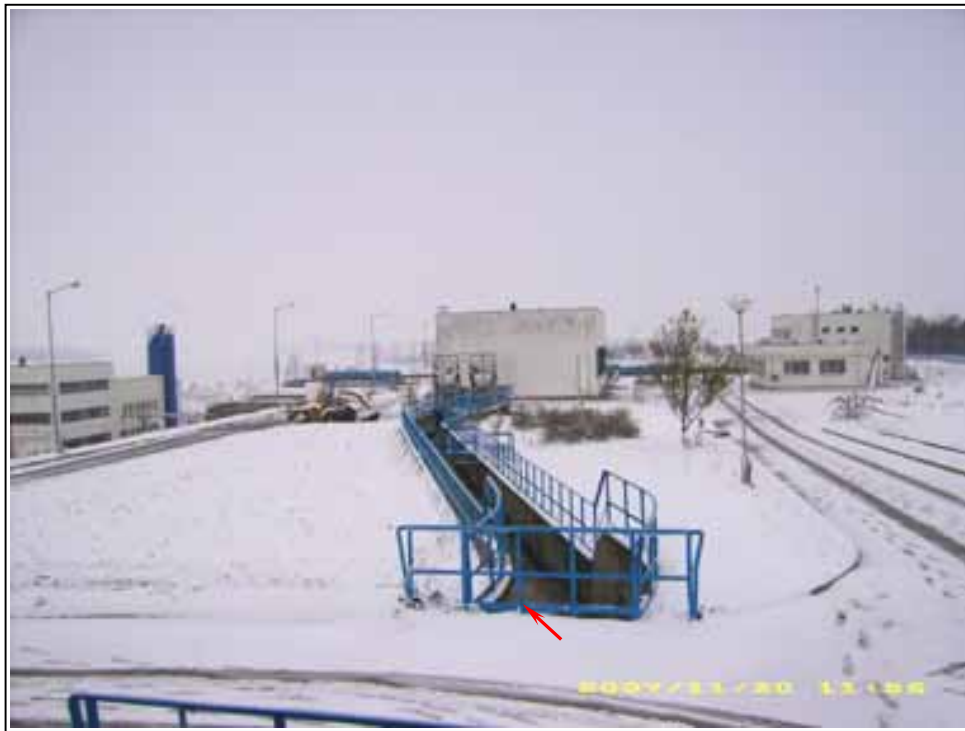
Pic.9 - Shumen WWTP: General view of inlet channel, racks and grit chamber
