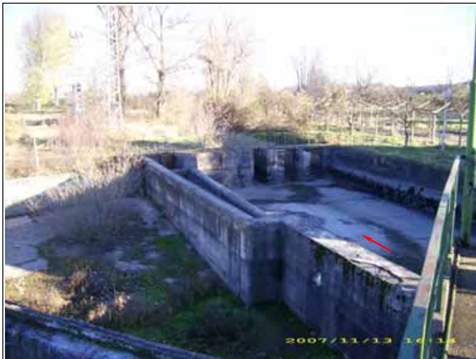
Pic.20 - General view of the intake chamber and the beginning of the Main Lower Right irrigation channel at Byala Cherkva weir
