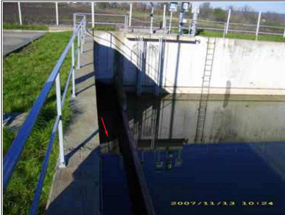
Pic.11 - Gorna Oryahovitsa WWTP: General view of inlet, inlet channel and storm water basin
