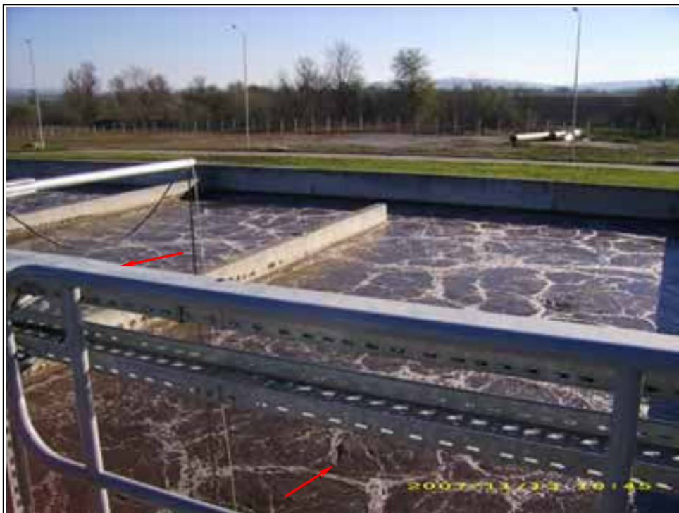
Pic.12 - Gorna Oryahovitsa WWTP: Aeration tank with nitrification, denitrification and phosphorous removal
