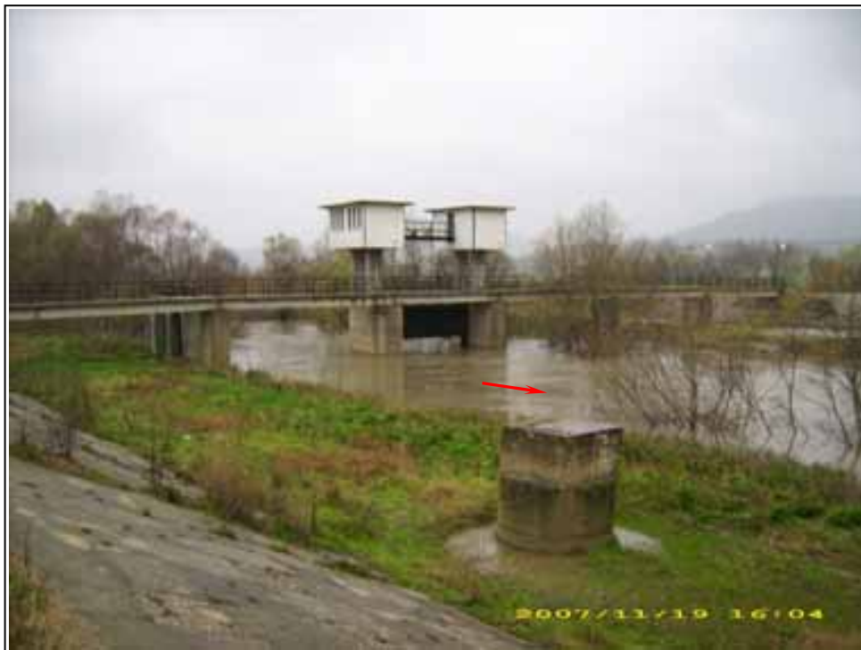
Pic.3 – General view of the bridge, the weir gate and the irrigation intake at Komunari village on the Golyama Kamchia River
