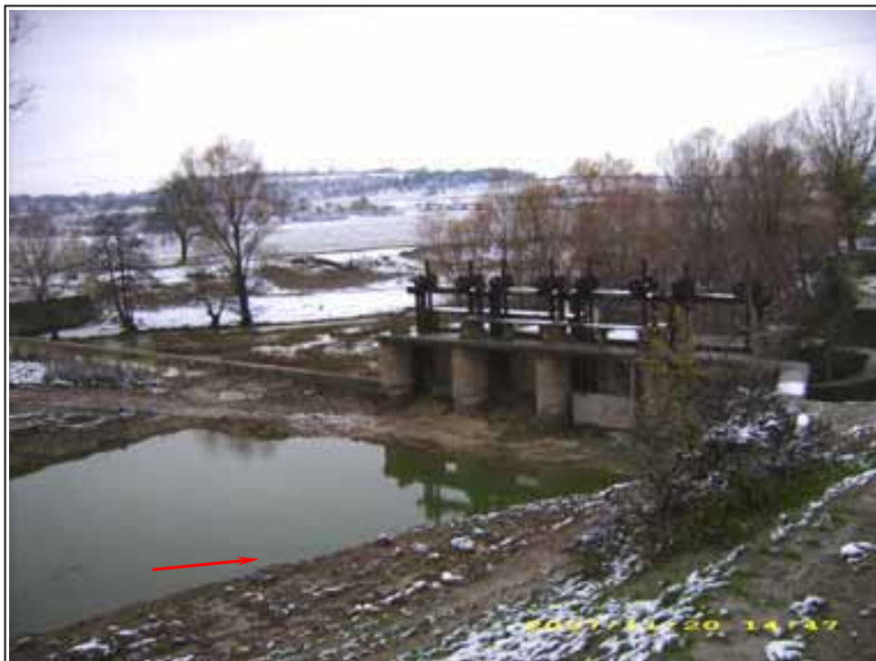
Pic.12 – The bridge and the gate mechanism of Ticha HPP water intake near Veliki Preslav town on the Golyama Kamchia River
