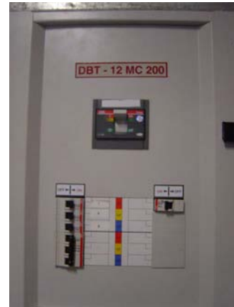
Switchboard installed at corridor
