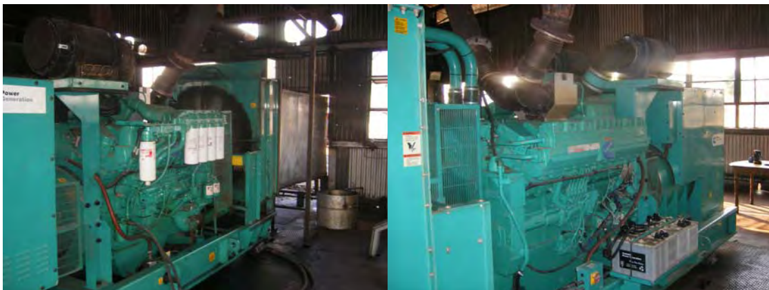
Fig.2.1 Mwinilunga Diesel Power Plant
