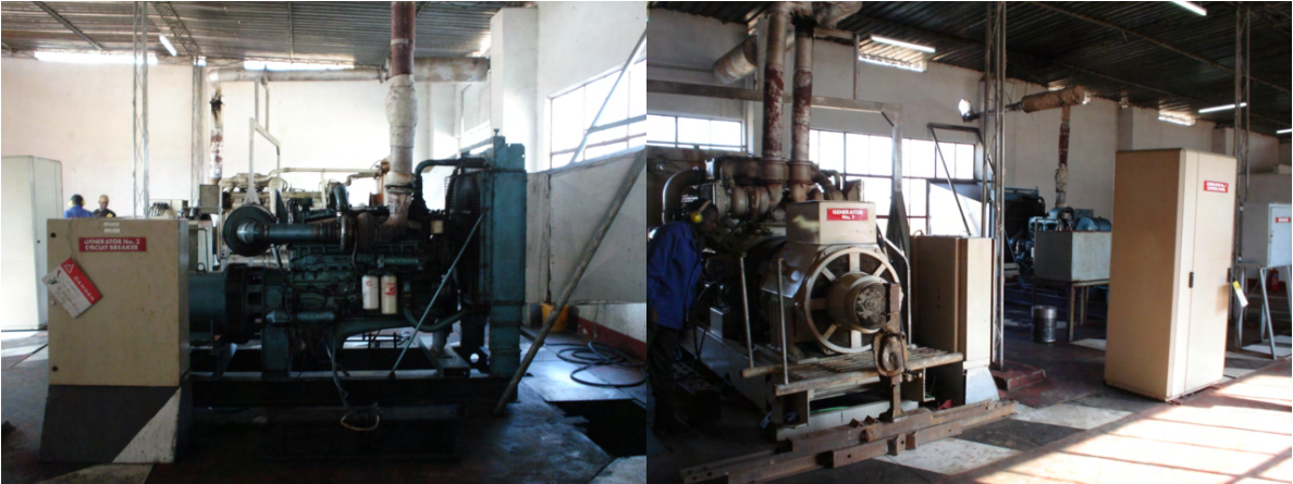
Fig.2.2 Chavuma Diesel Power Plant
