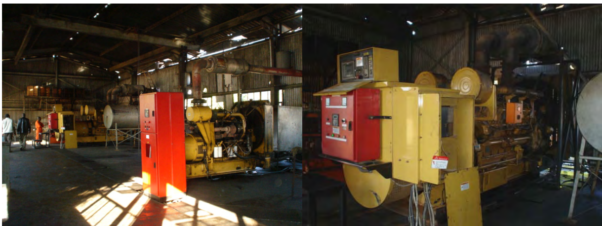
Fig.2.4 Kabompo Diesel Power Plant
