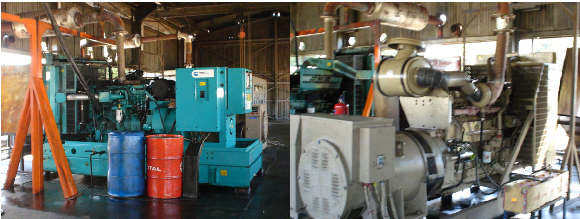
Fig.2.3 Zambezi Diesel Power Plant
