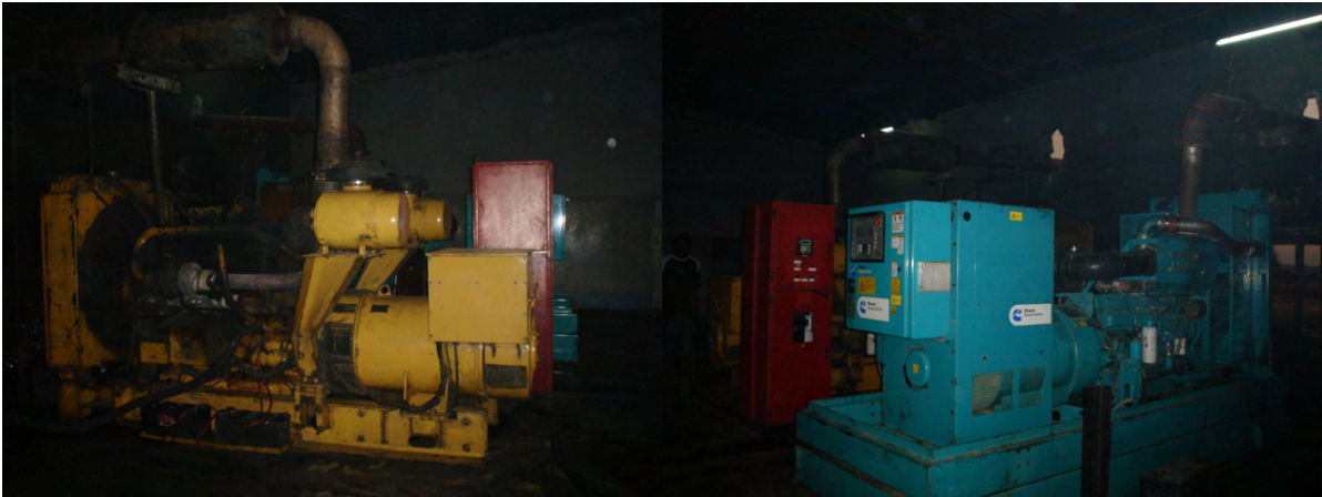
Fig.2.5 Mumfumbwe Diesel Power Plant
