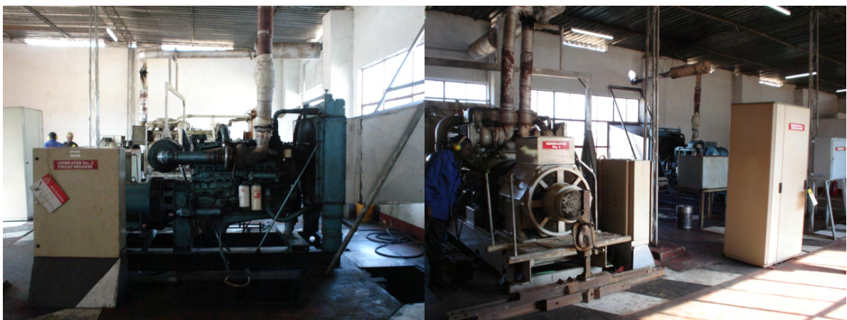
Fig.2.2 Chavuma Diesel Power Plant
