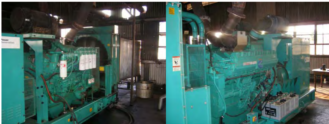
Fig.2.1 Mwinilunga Diesel Power Plant
