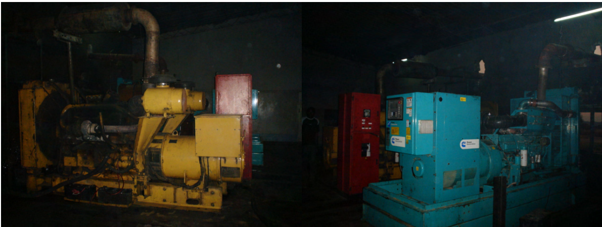
Fig.2.5 Mumfumbwe Diesel Power Plant
