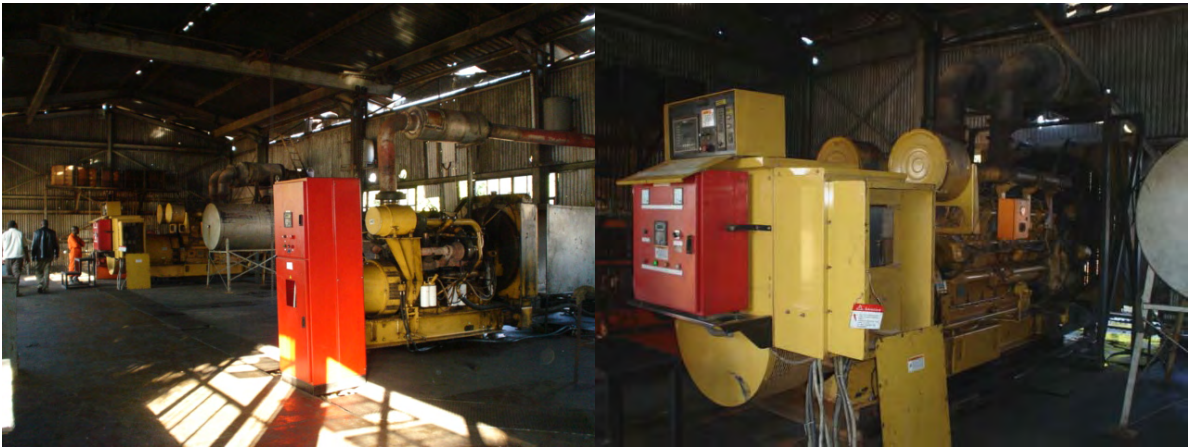
Fig.2.4 Kabompo Diesel Power Plant
