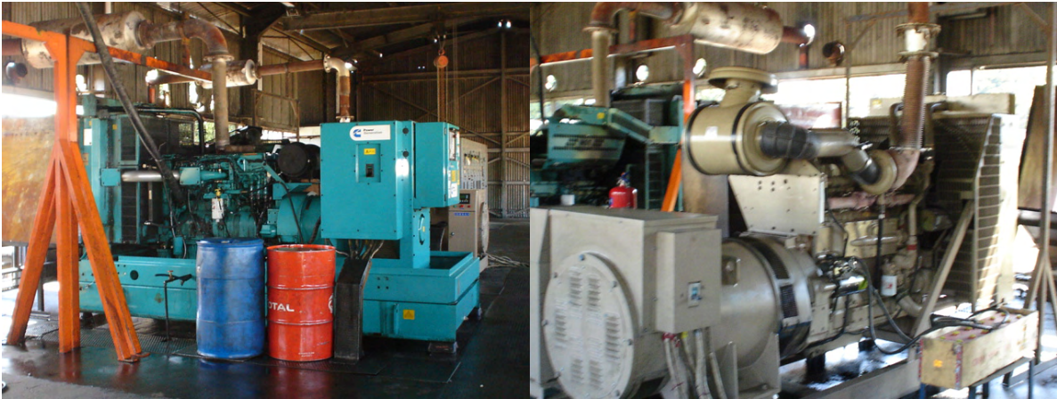
Fig.2.3 Zambezi Diesel Power Plant
