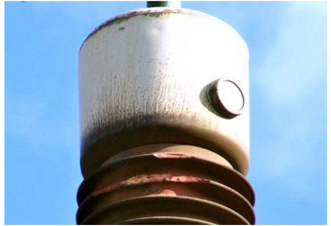
Figure 9 Chipped and Rusted Porcelain
