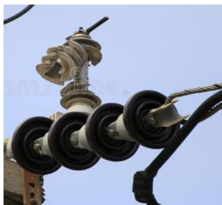
Figure 15 Cracked Lightning Arrester
