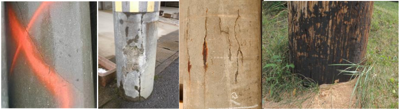
Figure 3 Cracked Electrical Poles
