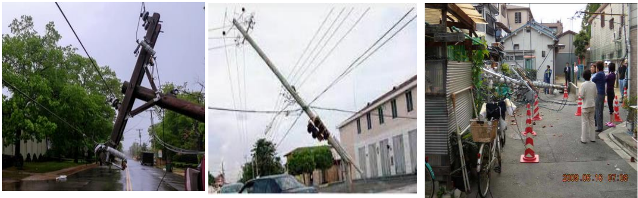
Figure 4 Falling Poles due to unattended cracks
