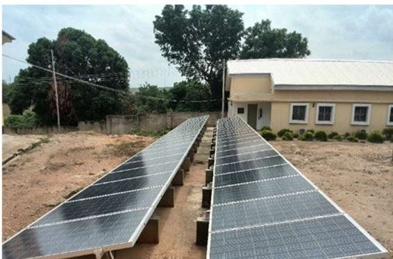
Figure 1.6. 10kW Photovoltaic Plant at Kainji
