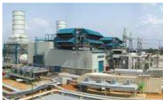
Figure 1.8. Afam VI Gas Power Plant.
