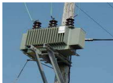
Figure 1.11. POLE Mounted Transformer.
