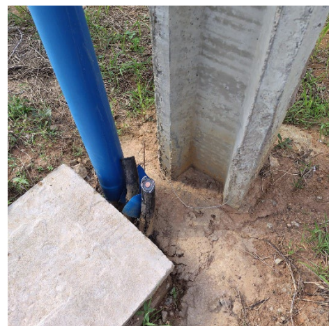
Figure 2-1-2.6 Theft Location at Cable Standing Part
