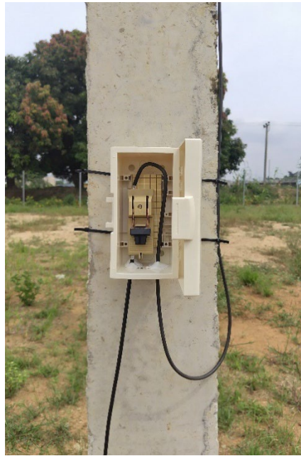
Figure 2-1-3-2.2 Breaker of Fault point
