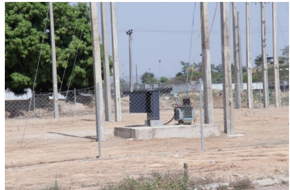
Figure 2-1-2.4 Distribution Transformer and Feeder Pillar
