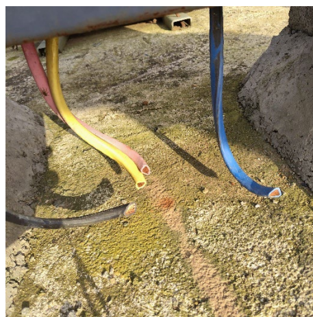
Figure 2-1-2.8 Theft Location of Cable Connecting Distribution Transformer and Feeder Pillar
