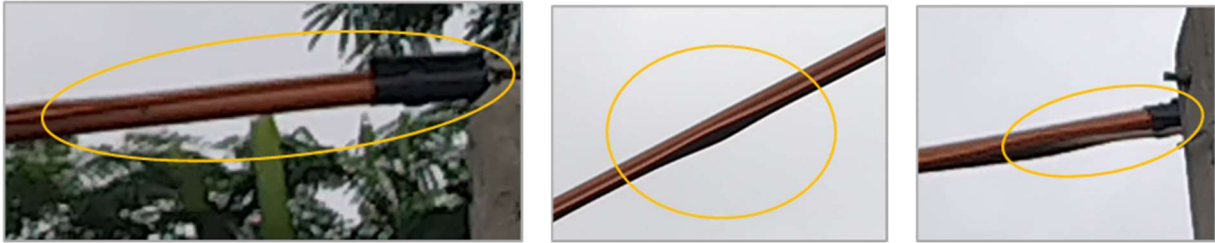
Figure 8 Defective construction confirmed
