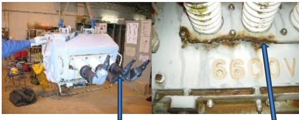
Figure 14 Cracked and rusted body which is a potential point of water ingress into the switchgear
