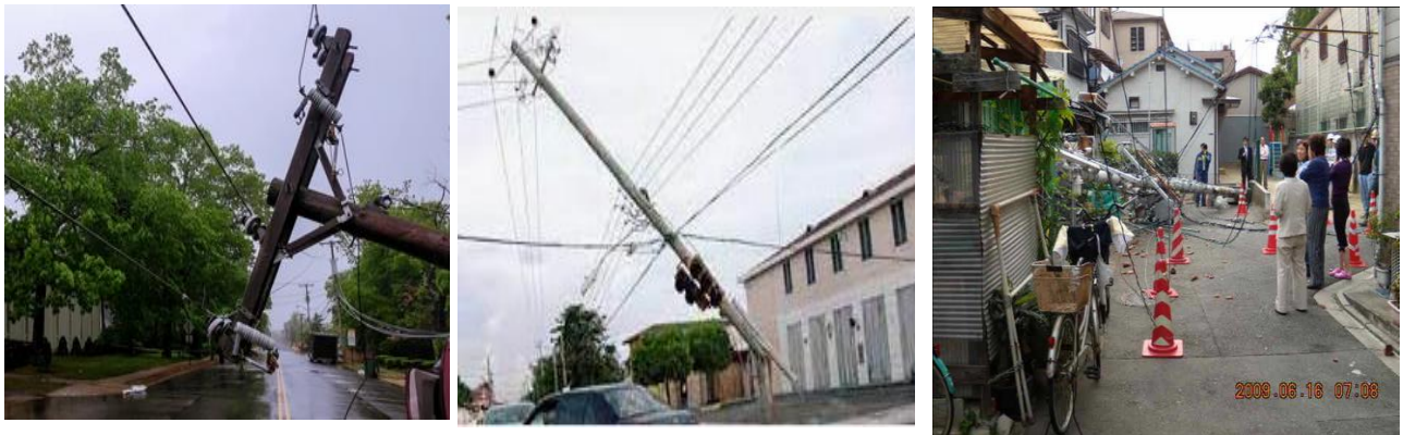
Figure 4 Falling Poles due to unattended cracks
