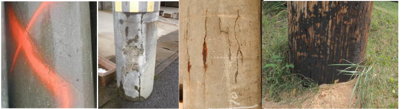
Figure 3 Cracked Electrical Poles
