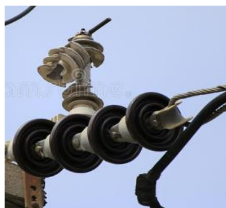
Figure 15 Cracked Lightning Arrester
