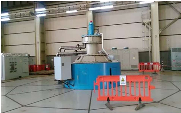
Figure 1.4. Refurbished 1G6 (120MW) at Kainji
