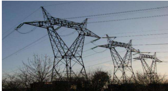
Figure 1.9. Transmission Power Lines.
