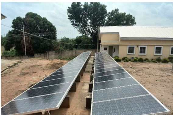
Figure 1.6. 10kW Photovoltaic Plant at Kainji
