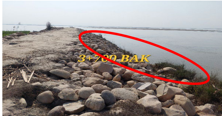
Damaged apron of the spur
