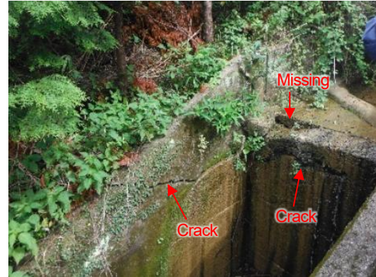
Cracks and missing in drop work
