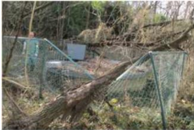
Deformation of safety fence
