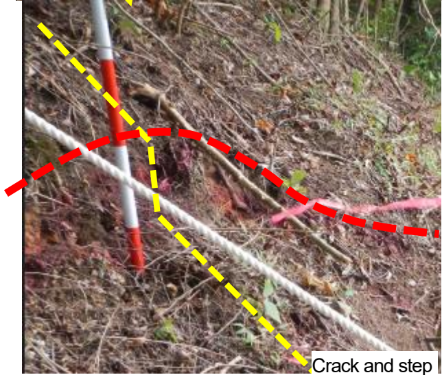
Figure 28 Image drawing and case study photo of facility deformation caused by slope activity
