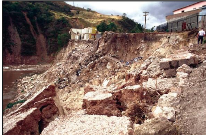
Figure 4 Landslide in the Mira Mesi neighbourhood, adjacent to the Choluteca River (AMDC)
