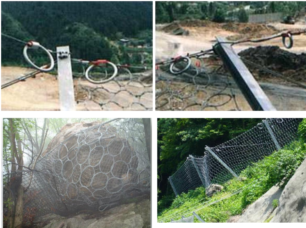
Figure 80 Case study of high energy absorption type rockfall protection fence work in Japan
