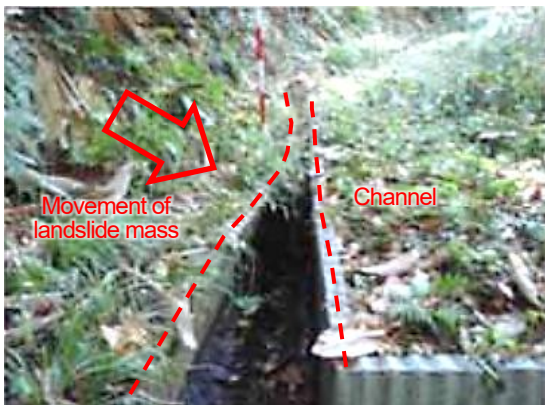
Channel deformation due to movement of landslide mass
