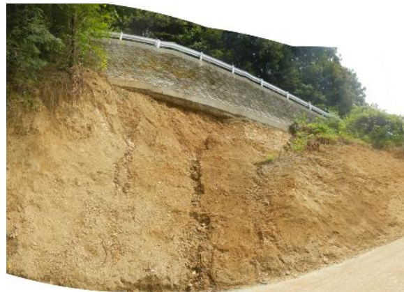
Foundation ground is eroded
