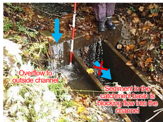
Overflow due to blockage
