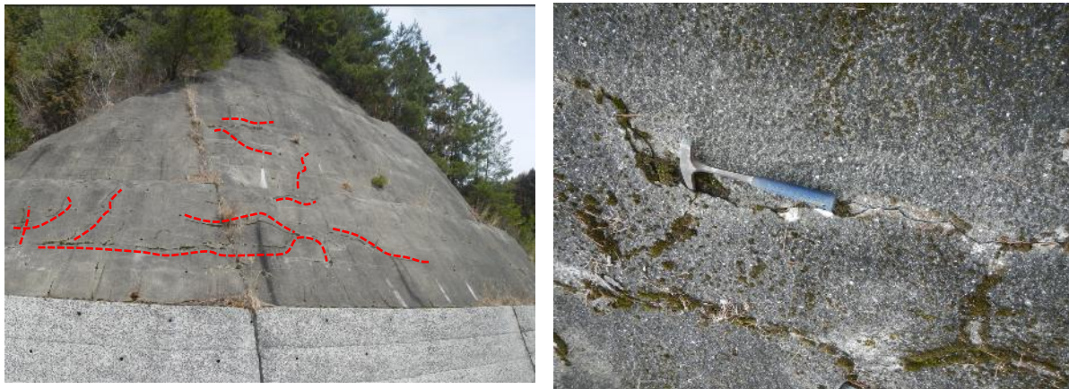
Figure 25 Case study photo of crack
