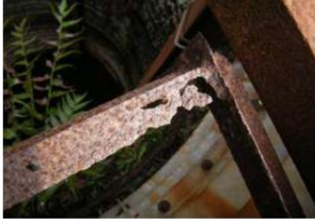
Deterioration due to rust (ladder)
