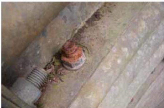
Corrosion of bolt
