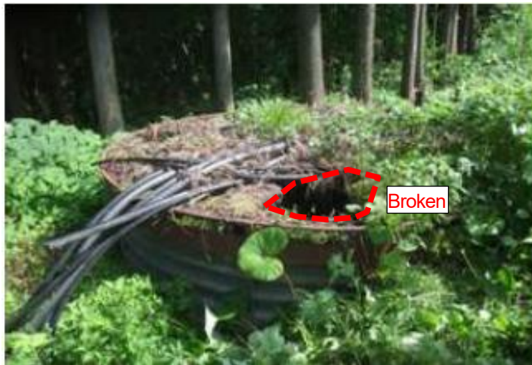
Deformation of canopy
