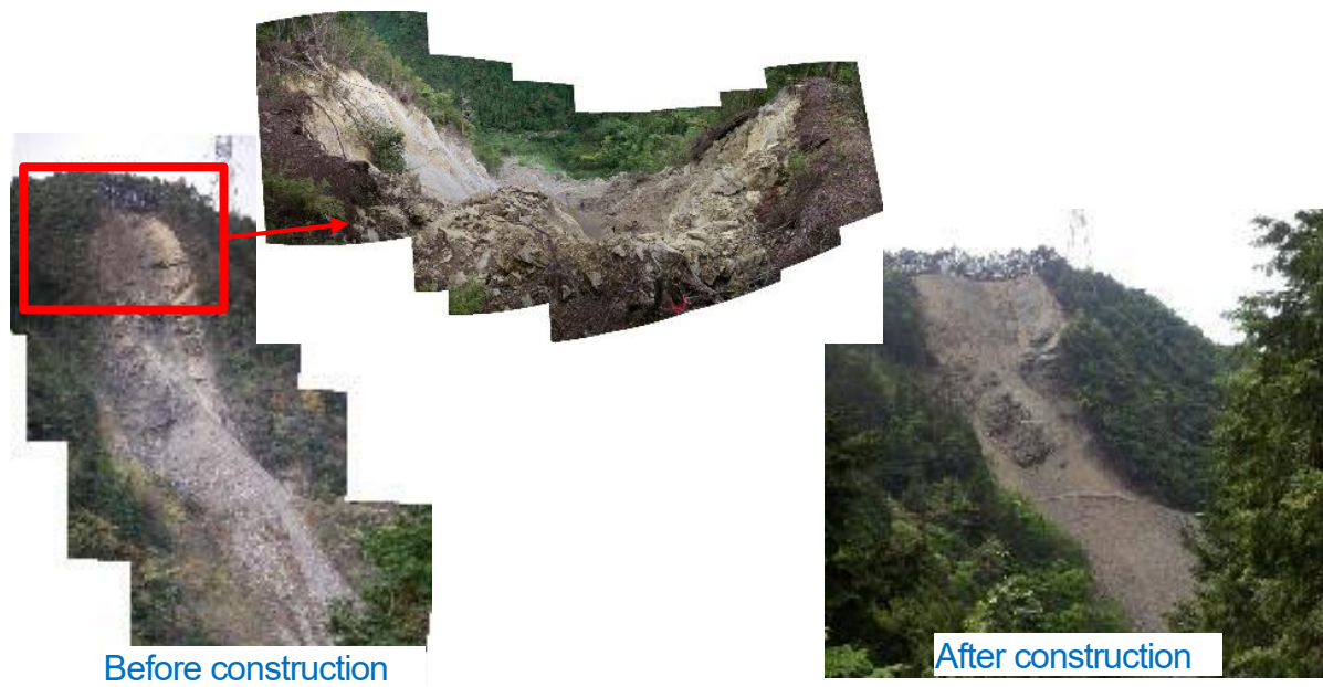
Figure 71 Case study of cutting slope work for unstable rock slope in Japan
