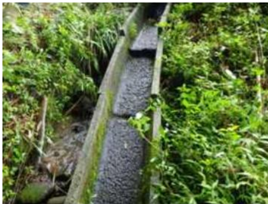
Subsidence and tilting in channel
