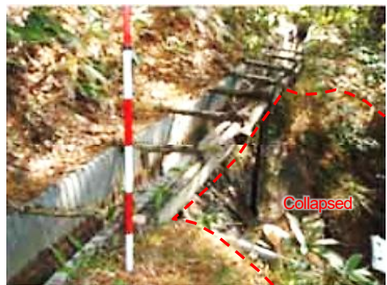
Slope collapse under channel
