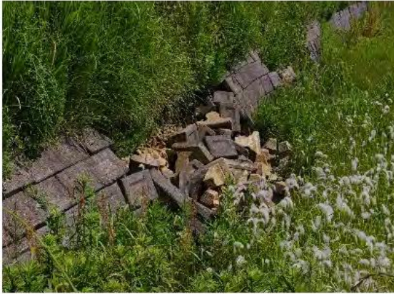
Collapsed concrete block masonry wall
