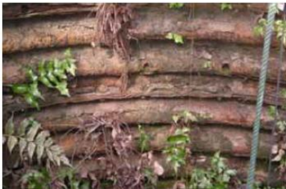
Corrosion of liner plate
