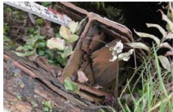
Corrosion of Vertical Stiffener
