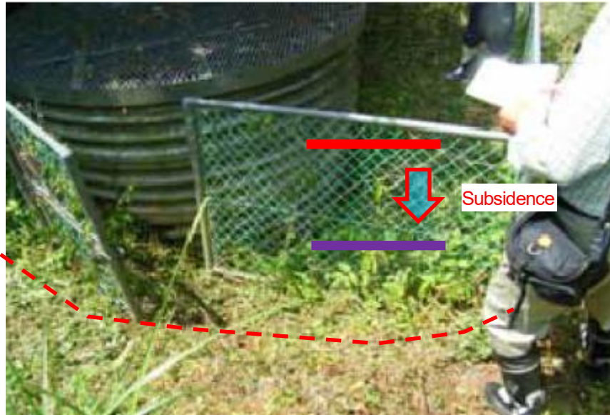
Subsidence of surface ground and deformation of safety fence
