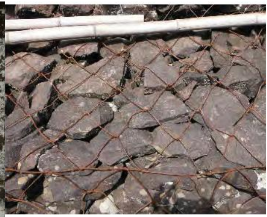
Rusted gabion frame
