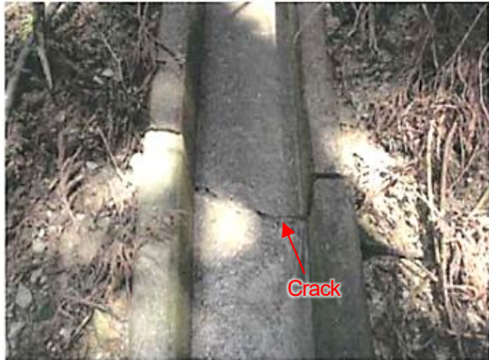
Crack in channel
