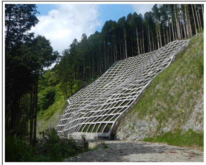
Figure 38 Case study photos of crib work
