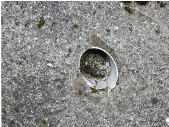
Figure 57 Clogging situation of drainage pipe.
