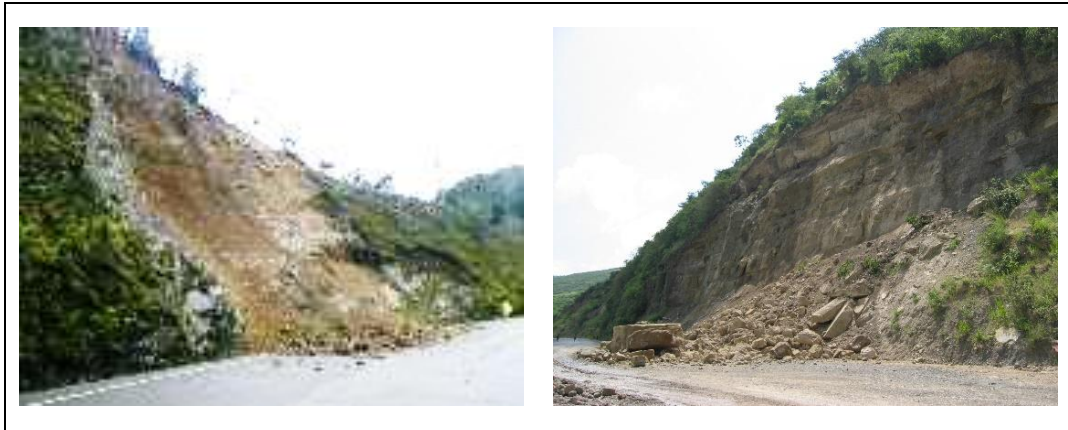
Figure 2.2 Slope failures in Ethiopia (JET)
