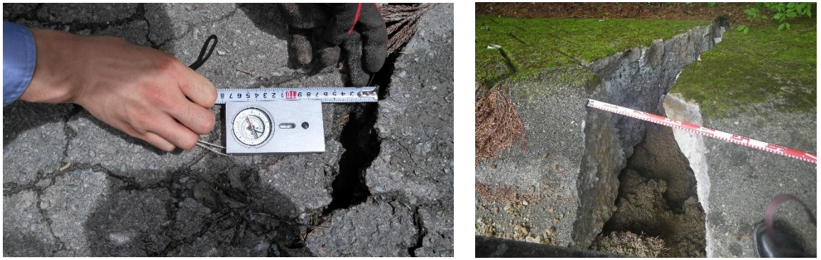
Figure 1.2 Measurement of Crack (JET)
