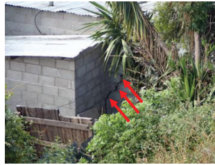
Crack on the wall
