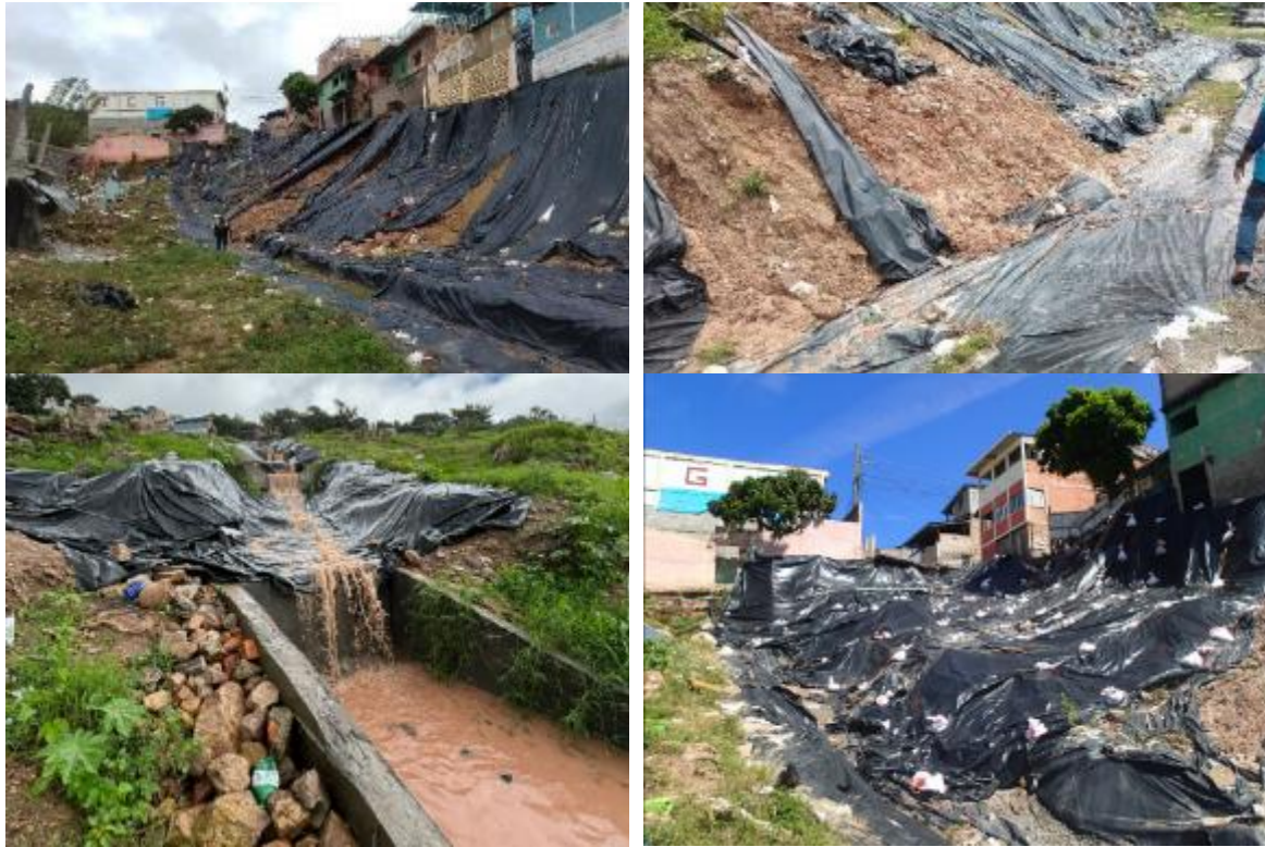
Figure 145 Monitoring and maintenance situation
