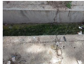
Cracks in drainage
