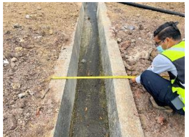
Channel size measuring situation
