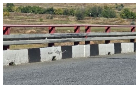
Photo 1-2-14 Scratch Marks on the Guardrail of the Naryn River Bridge
