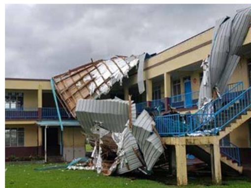
Fig. 4 Bhawani Dayal Arya College Sustained Extensive Damage from Tornado
