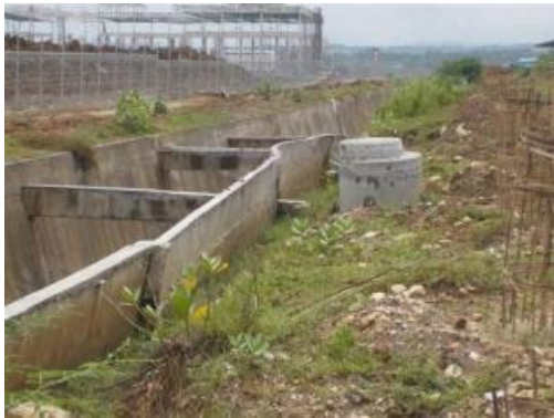
(a) Damage to drainage facilities (Indonesia)
