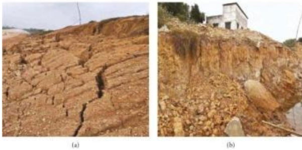
FIGURE 1: Cracking and collapse of expansive soil slopes.
