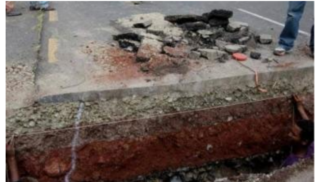
Source: Evaluation of Damage to a Road and Sports Complex on Expansive Clays , M. B. Mgangira, P. Paige-Green (2008).
