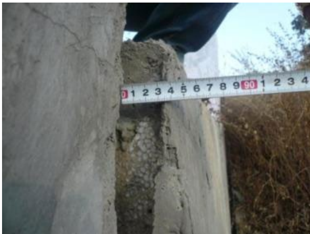
(c) Deformation due to swelling pressure on the culvert sidewall of road embankment (India) - Dry season
