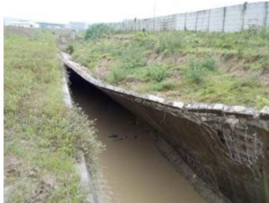
(b) Damage to drainage facilities (Indonesia)
