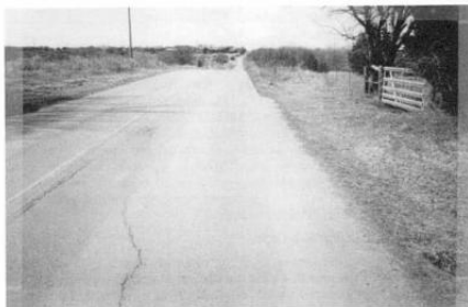
a. Photograph looking west showing cracks in westbound lane and proximity of Chinese Elm tree
