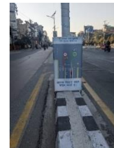
Installed in the median strip
