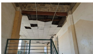
Ceiling blown away
