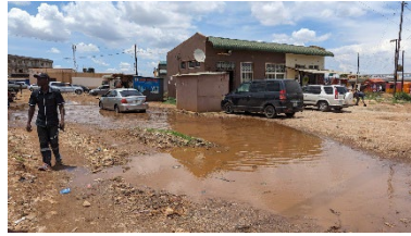
Drainage system is weak and frontage road at entrance is not paved.
