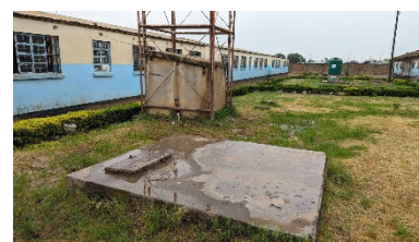
Leakage of water tank
