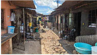
Pavement is deteriorated and repaired with blocks.
