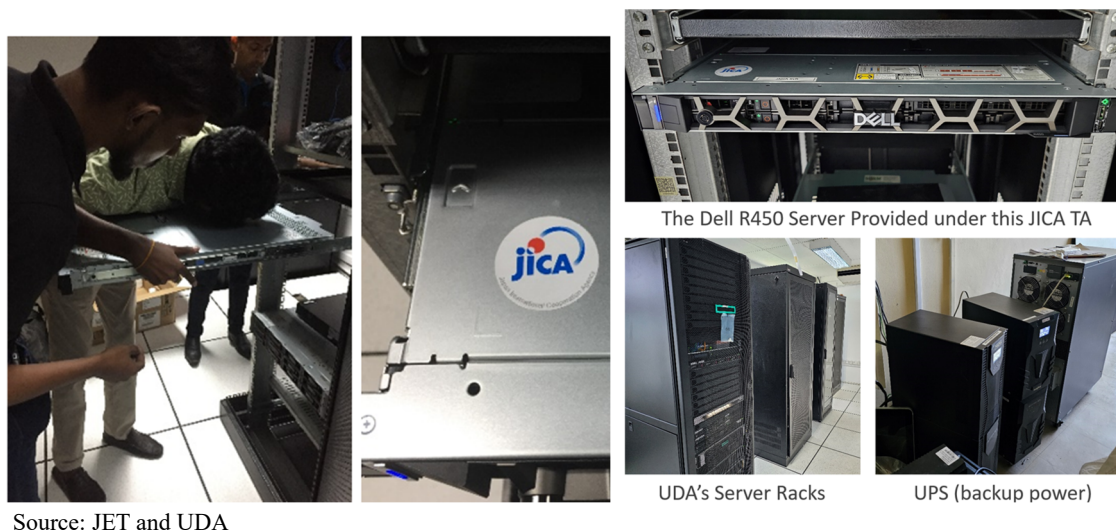
Figure 3: Server installed in UDA
