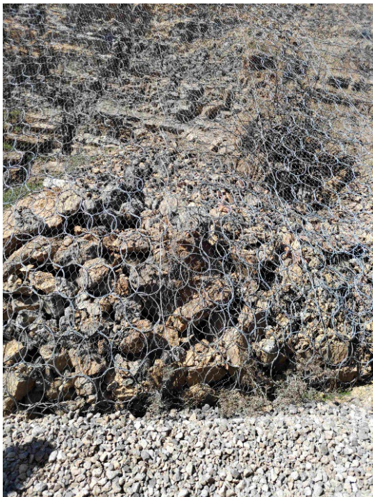
The diameter is small, but the frequency of falling rocks is high
