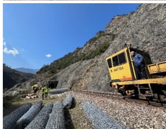
Figure 2-9 Rock Fall Protection Wire Mesh Constructed by TCDD
