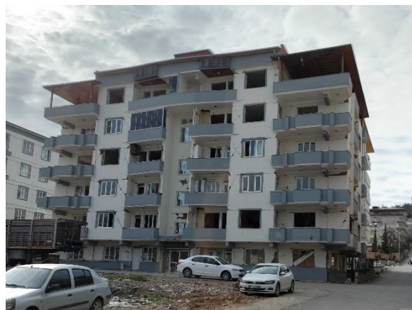
Figure 6-8 Building With Damage Due to the Earthquake
