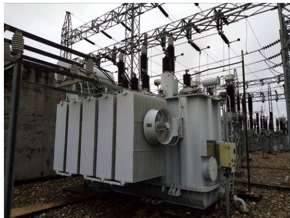
Figure 5-2 Failed 115/22 kV Transformer No.2 (Taken by JICA Expert Team)
