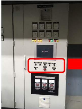
Overall view of direct control panel
