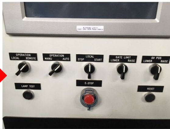
Enlarged view of the switches for direct operation
