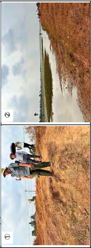
Embankment of Kpob Trobek Dam. It has been heavily eroded even though MOWRAM rehabilitated in 2022. In the flood season, the water level sometimes reaches almost the same level of the top of embankment, which implies the lack of discharge capacity.
