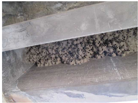
Photo 4-10 Nest and dropping of birds is a problem for bridge maintenance
