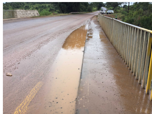
Photo 4-6 Ponding Water and Mud on the Deck
