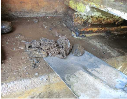
Photo 4-8 Mud, Debris & Sand on Bearing
