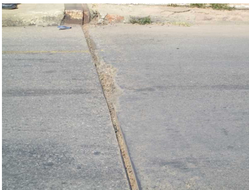
Photo 4-5 Joint is Clogged with Sand and dirt
