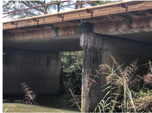
Photo 4-16 Tree Hanging Over the Girder
