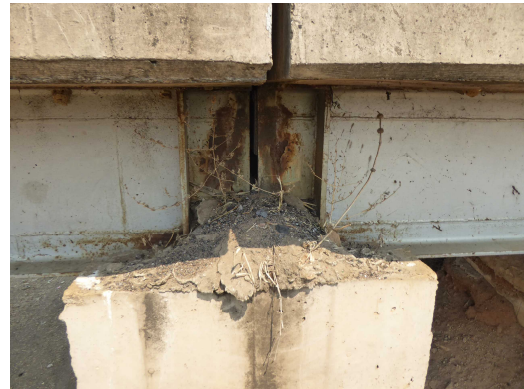
Photo 4-4 Vegetation and Soil on the Girder
