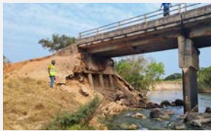
Fig 3. Eroded protection works on the bridge abutment
