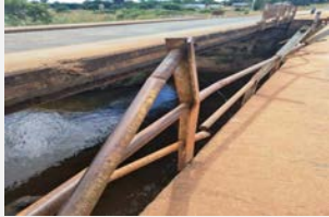
Fig 1. Damaged railings/ rusting on the steel members
