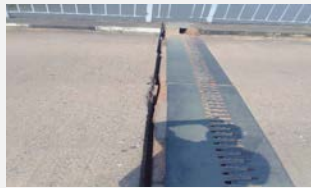
Fig 4. Damaged expansion joint
