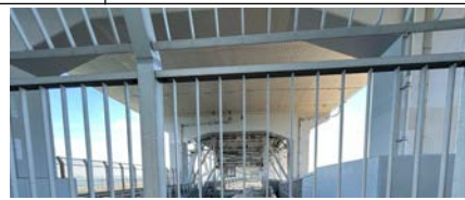
Cathodic Protection using Titanium ribbon mesh anodes (Electric Power Supply)
