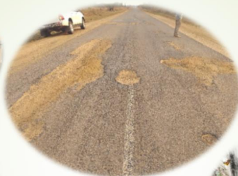
Potholes on M8 Road
