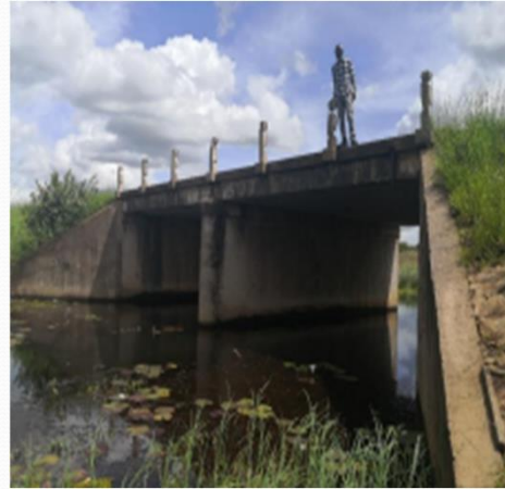
Discovering of serious damage result in high repair cost
