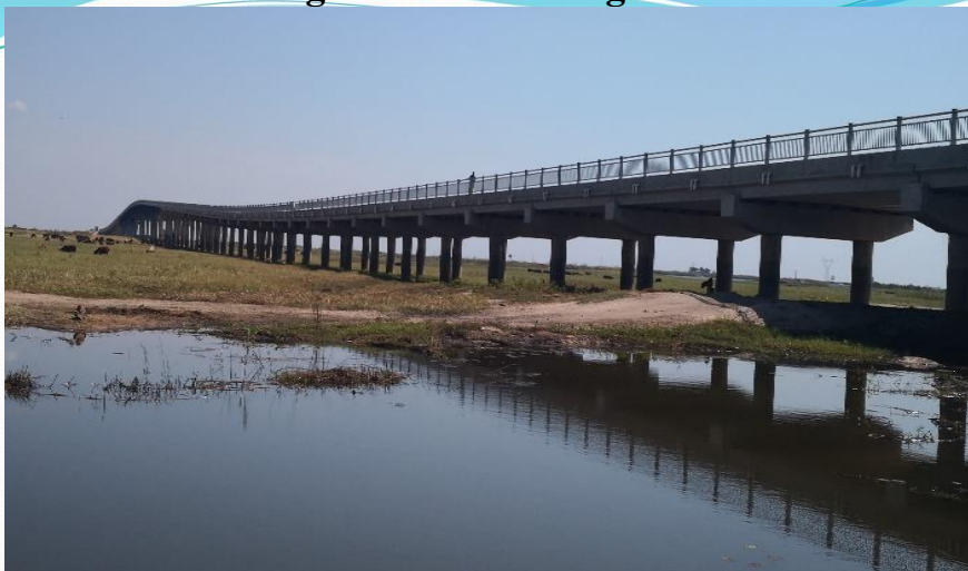
Timely Routine and Periodic Maintenance of bridges will result in reduced cost of maintenance and prolong life span of bridges
