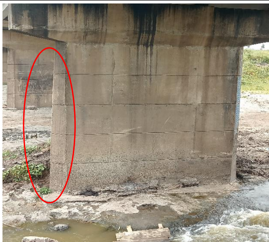
The shape of the pier was considered for the impact of the water
