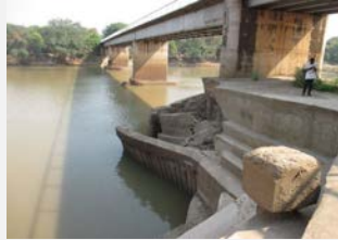
Fig 2. Eroded protection works on the bridge abutment
