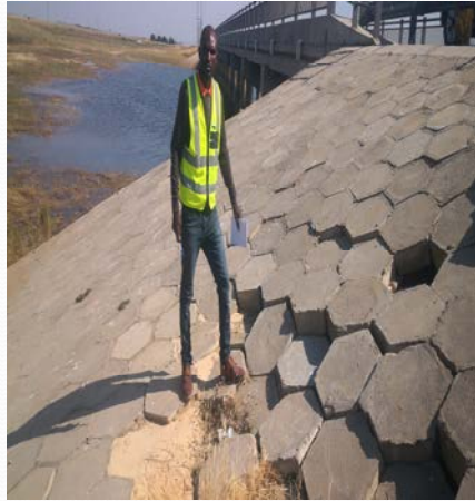
Repair of minor damages result in simple repair low cost
