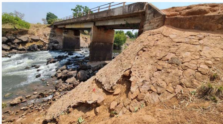
Damage due to delayed Maintenance of the Bridge
