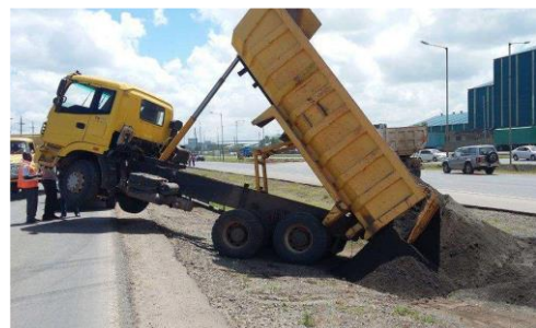
Tampering with overload evidence
