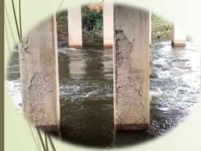
Spalling on Concrete Piers
