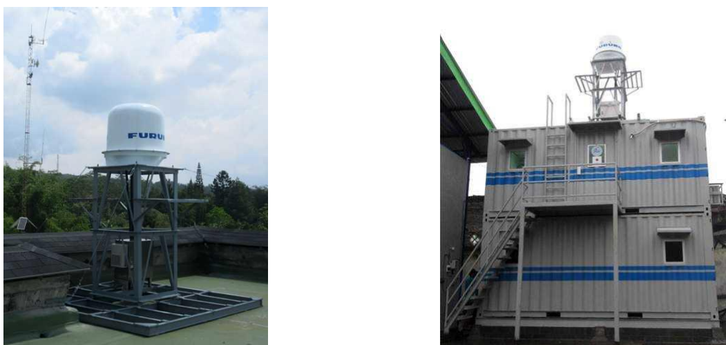
Figure 2-5 Condition of the X-band radar installation
