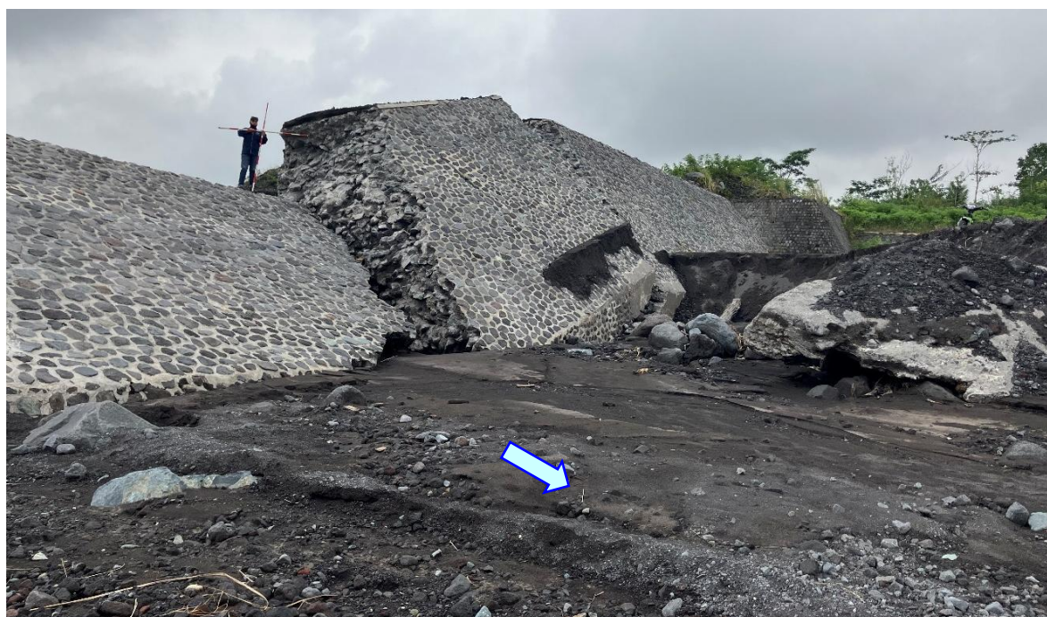
Figure 3-56 Damage to the left wing of DD Leprak 2 (May 2024)
