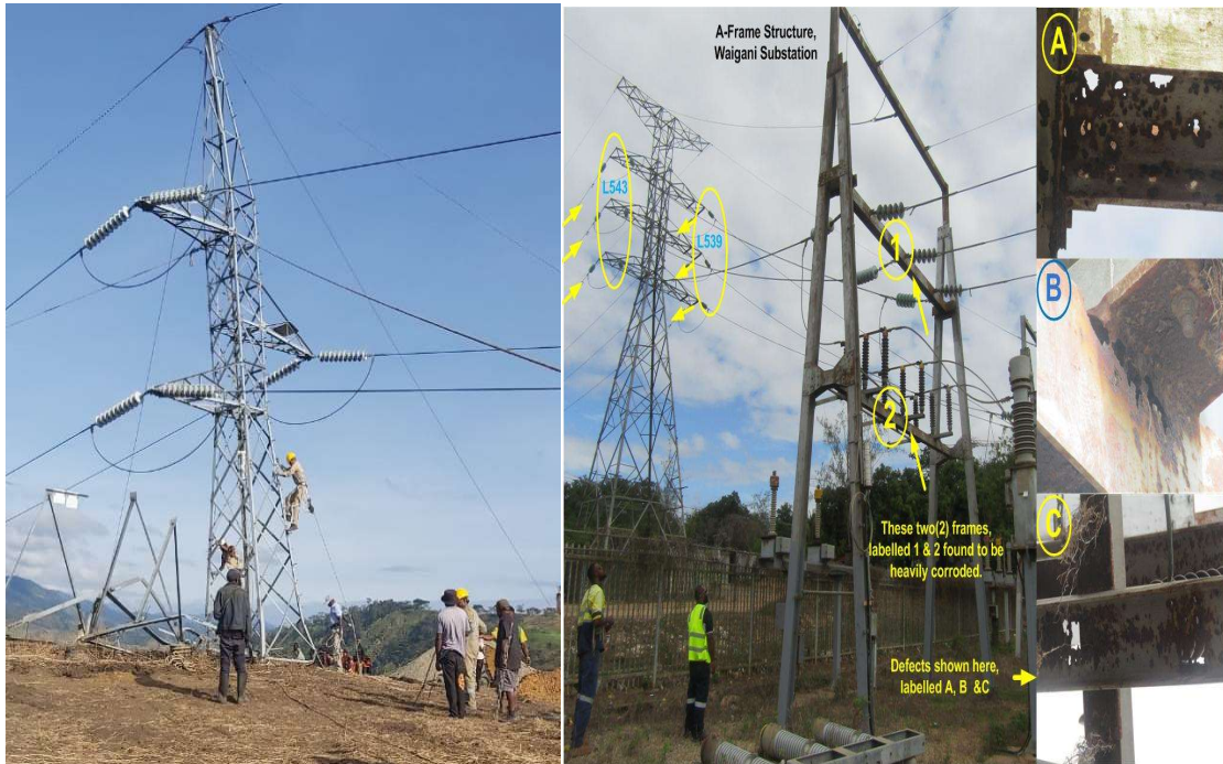
Fig1. The steel tower was collapsed in L602 Fig2. The gantry is being corroded in Waigani substation
