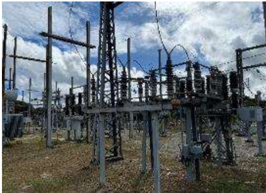
Figure.1 Line arrester for the leakage current measurement training (Boroko substation)
