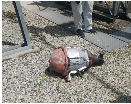
3. Collapsed circuit breaker part in Rouna2 Sub.
