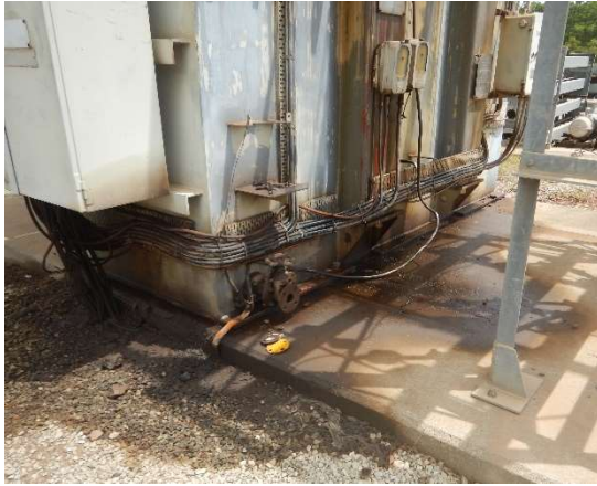
2. Oil leakage from Trans. in Waigani Sub.
