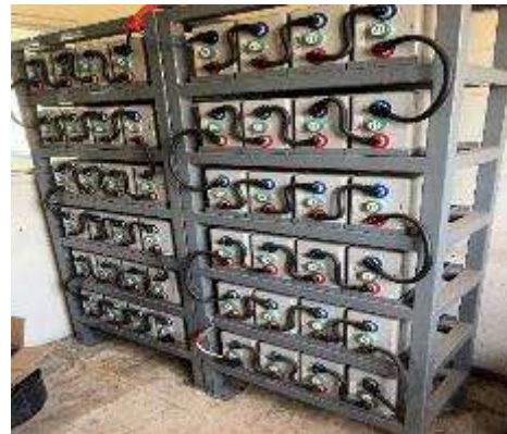
Figure 2 Batteries for the battery tester training (Boroko substation)
