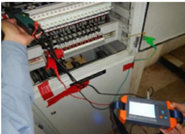
Training for DC Earth Fault Locator (WG2-2)
