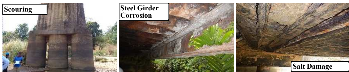
Figure 2-2 Major Deterioration of Bridges
