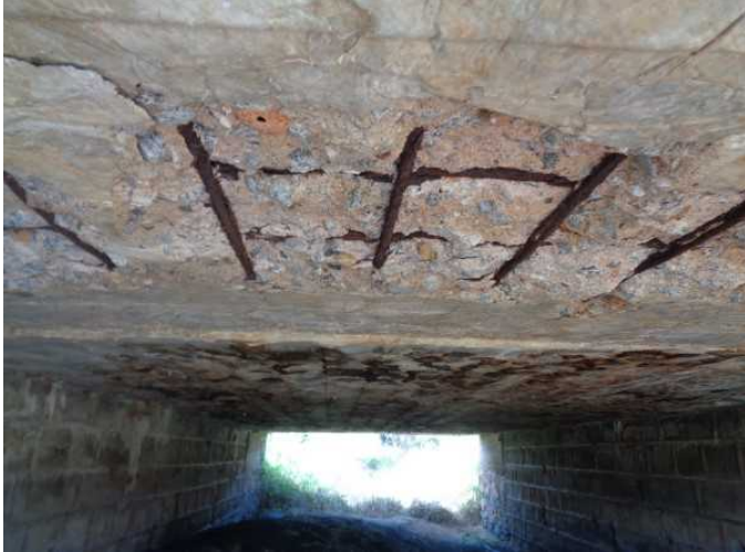
Deck reinforcement badly exposed
