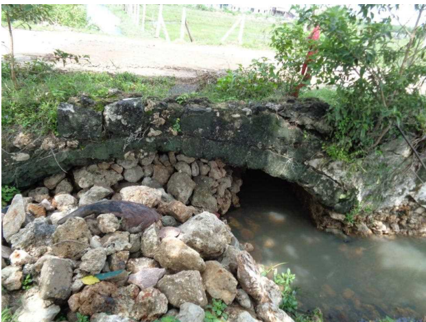
Existing arch bridge collapsed, temporary arrangement with boulder fill
