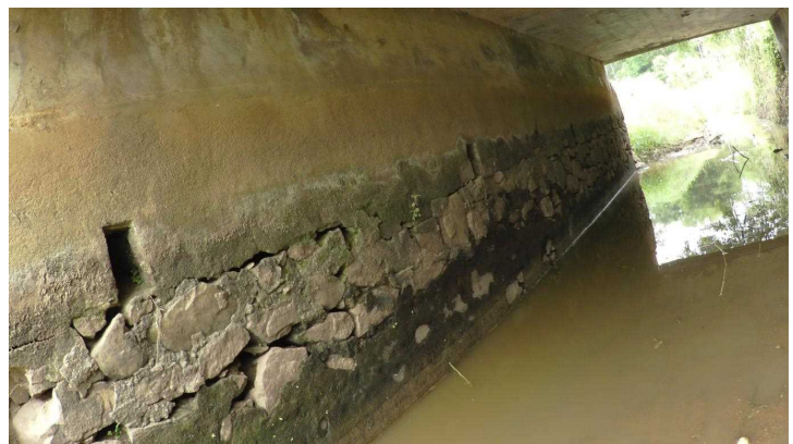
Weak abutment with loose boulders
