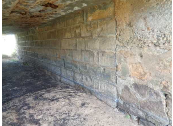
Deck reinforcement started to corrode
