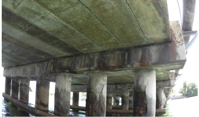
Badly damaged pier capping & pier columns with exposed reinforcement
