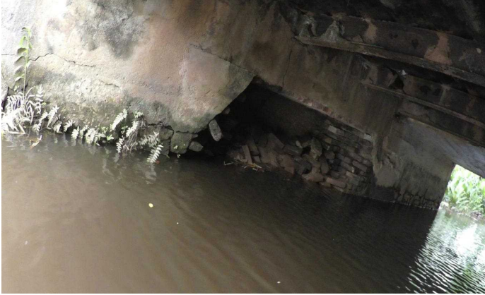
Weak abutment with loss of bricks
