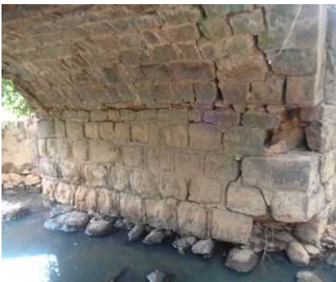
Cracks on arch barrel
