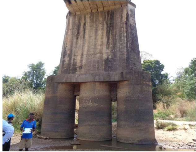
Badly scoured foundation
