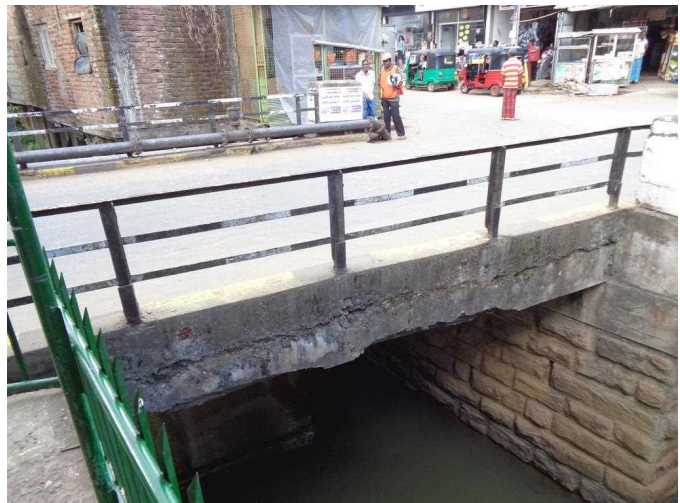
Reinforcement exposed in deck
