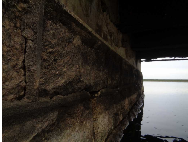
Very badly corroded RSJ & weak abutment
