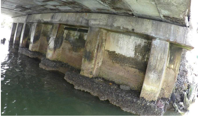
Collapsed wingwall, PSC beam reinforcement exposed
