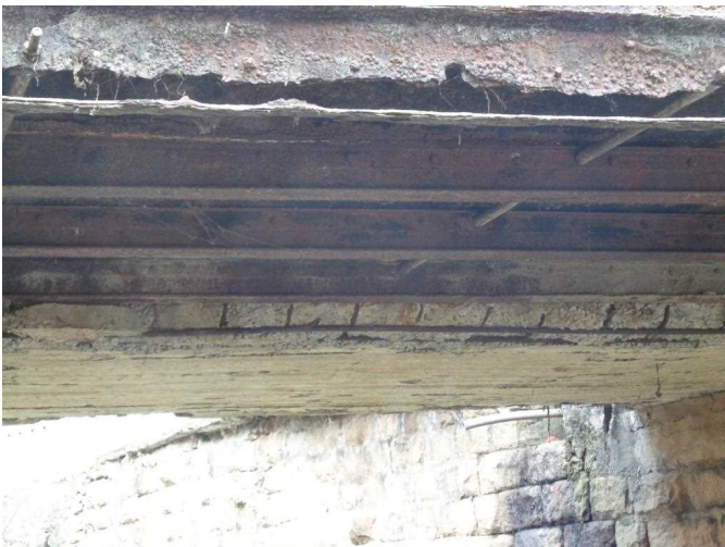
Very badly corroded RSJ
