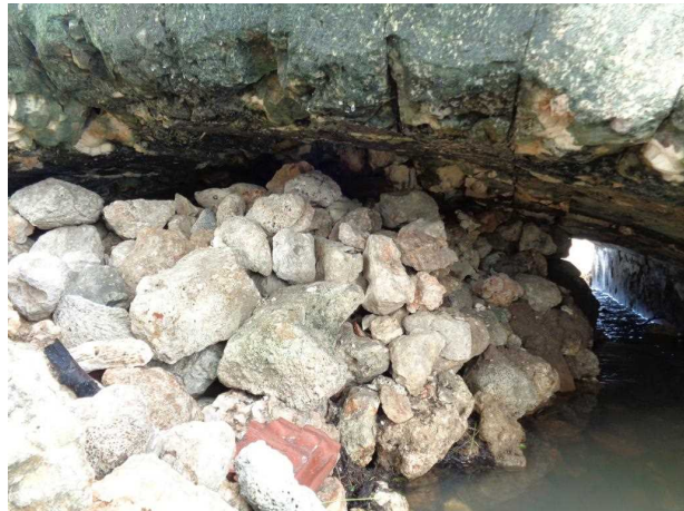
Waterway is filled by boulders
