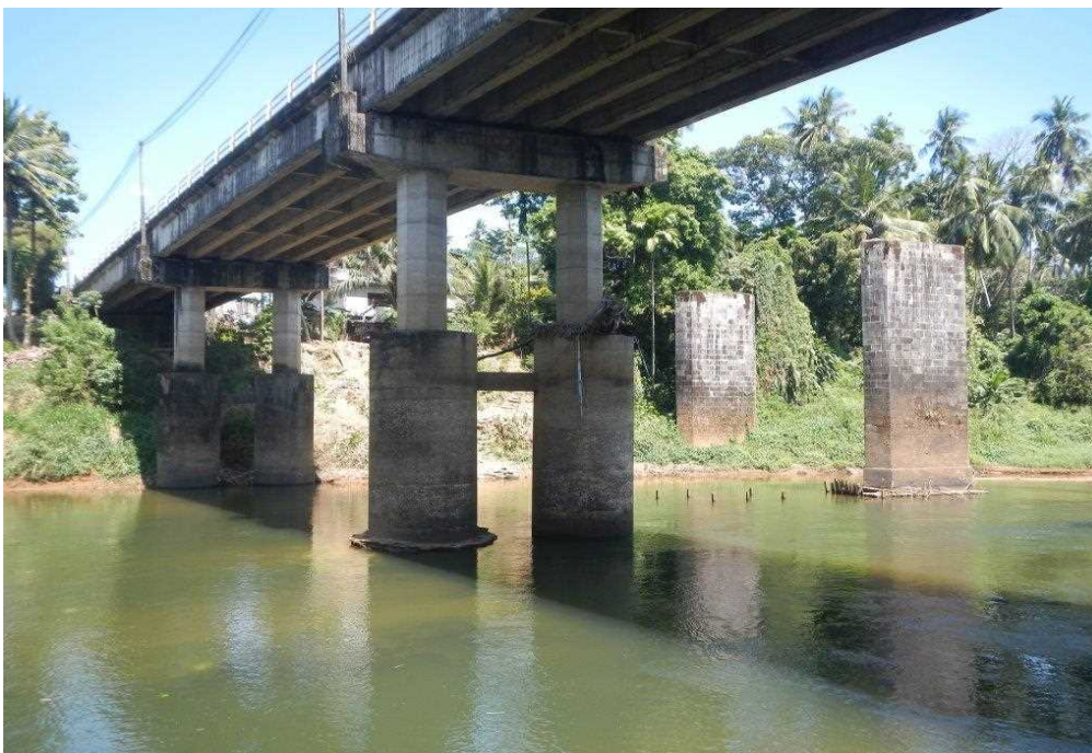
Badly scoured foundation
