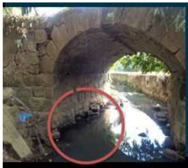
Foundation is scoured
