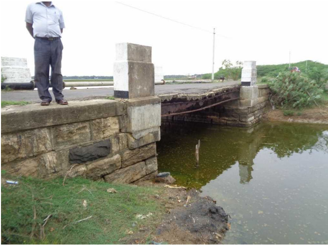
Very badly corroded RSJ
