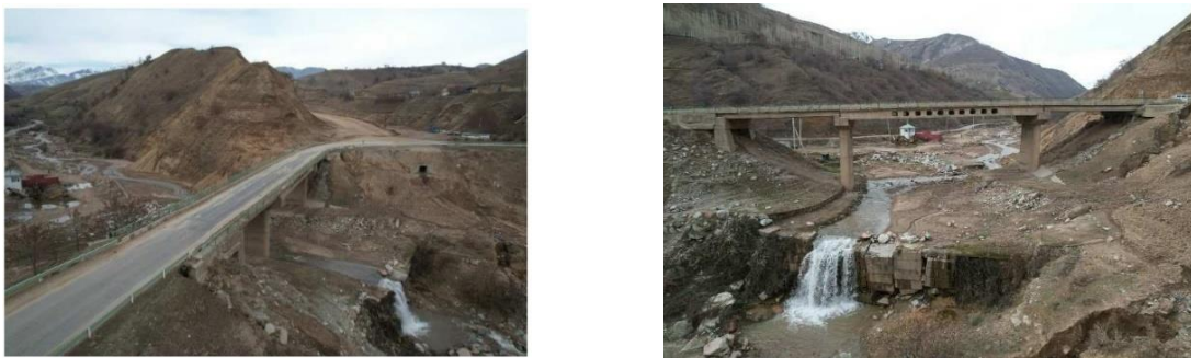
Figure 2-19 Aerial View of the Bridge Taken by Drone Provided in the Project
