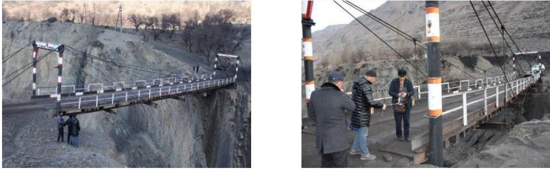
Figure 2-20 Inspection of the Damaged Bridge under Sughd SETM Jurisdiction
