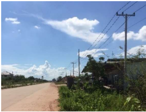
22 KV Electric Line
