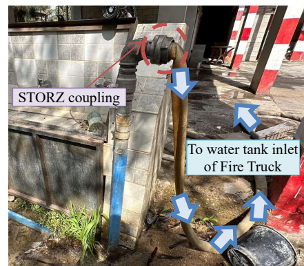
Photo 2-1 Fire Hydrant at a CDC
