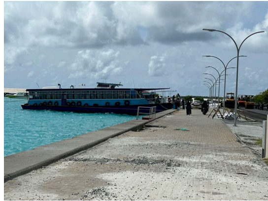
Situation of Apron Subsidence
