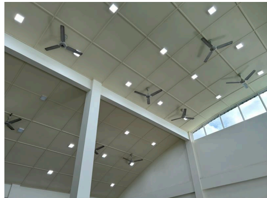
Terminal Ceiling (blower fan)
