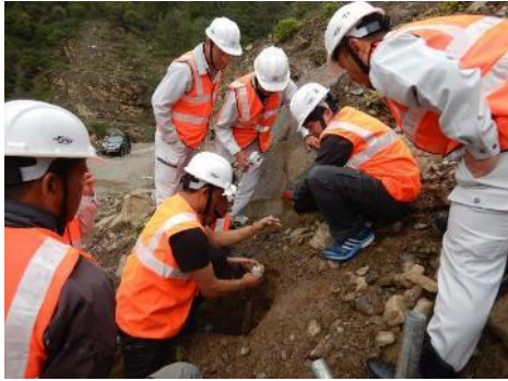
Output 1: First seminar Explanation of how to install monitoring equipment at construction site (4/17/2019)
