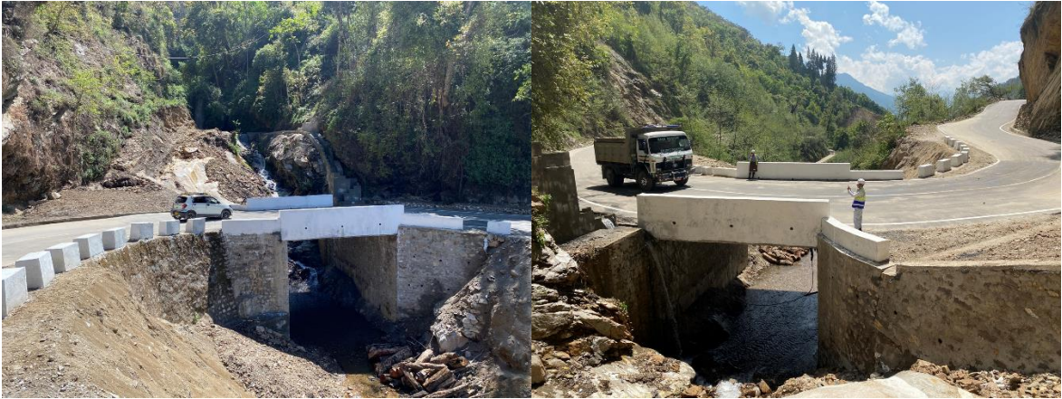
Overall view of the culvert after completion (left: from downstream, right: from upstream)
