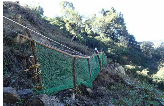
Temporary rock fall protection fence
