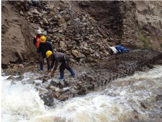
Damage to right bank foundation (Apr/19/2020)
