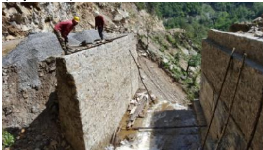
Damage to right bank foundation due to rising water (Jun/4/2020)
