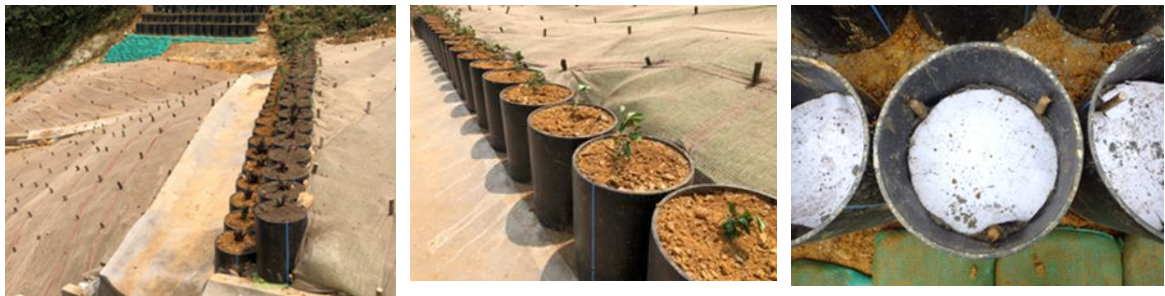
Pot planting (Berm drain 3, Y2) Row of vegetation pots 50 pots \times 56 pots (site of stepped drain: 3pots) (Source: JET)
