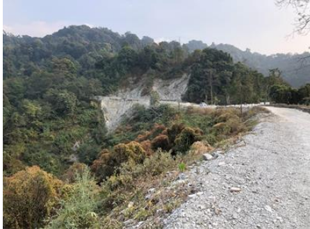
Photo 3.3-7 Distant view of the candidate slope (Road slope in front is unstable).
