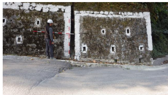
Photo 3.3-10 Settlement of the road on the east side of the slope.
