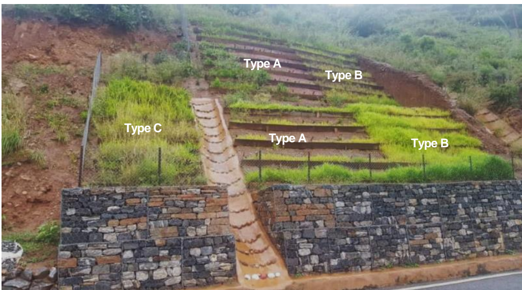
(Source: JET) Photo 3.3-31 Slope conditions about three months after vegetation construction (September 26, 2020)
