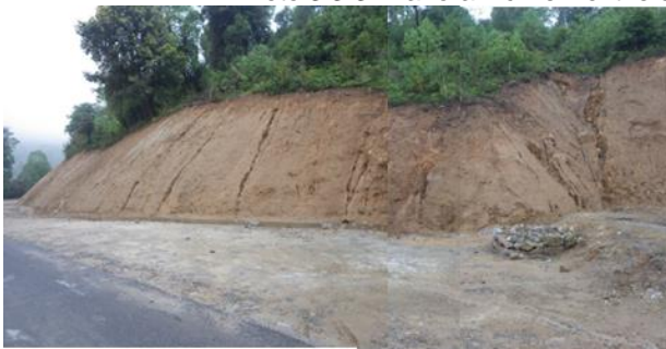
Photo 3.3-4 The one aspect of the slope with several gully erosion.
