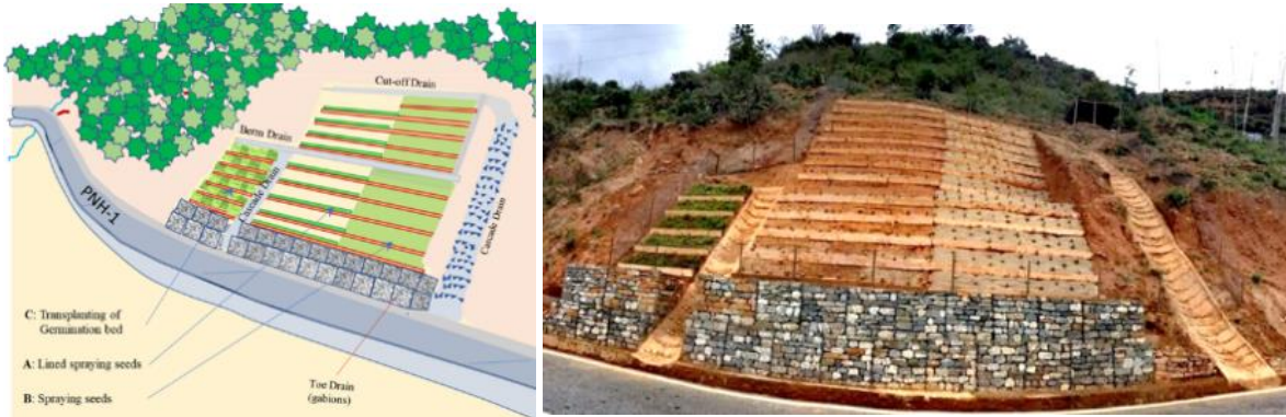
(Source: JET) Figure 3.3-29 Overall view of the project (left), slope immediately after vegetation construction (right) (May 31, 2020).
