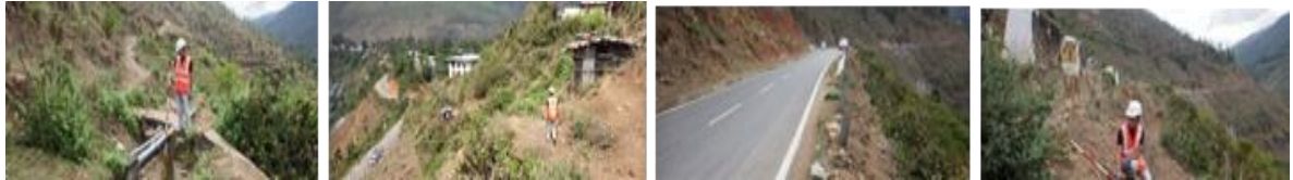
Upper path and waterway Slope and upper path seen from the east Road condition Road valley side slope (Source: JET)
