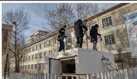
Installation of the PM sampler (23 November 2021)
