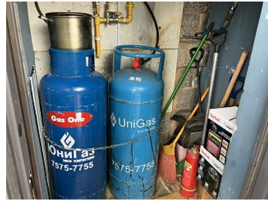
LP gas use in restaurants No metered management of the remaining gas, but one cylinder is alternatively replaced by the supplier on a regular schedule.
