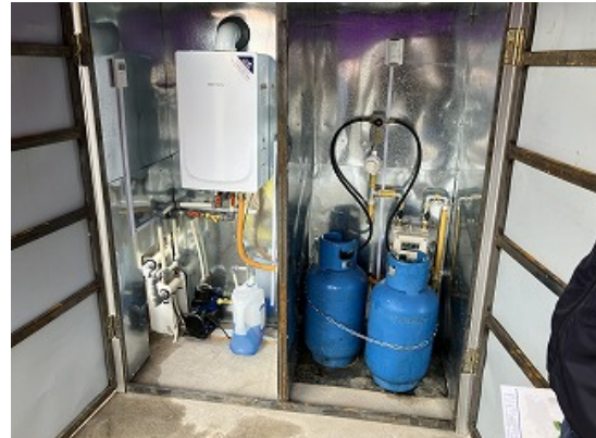
Gas hot water supply facility Divided into water heater and gas cylinder chamber; 14 kg cylinder used.
