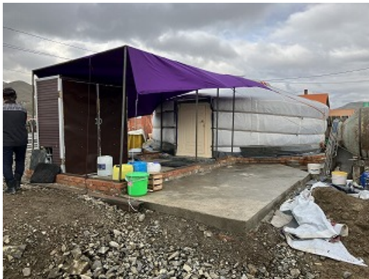
Ger with gas heating system (floor-heated) A gas hot water supply facility is connected to the traditional Ger.
