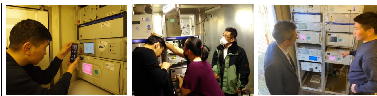
Photo 3-2-2 Operation and Maintenance of AQMS by DAAEP
