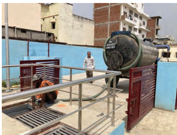
30KLD PSTU and septage receiving facility
