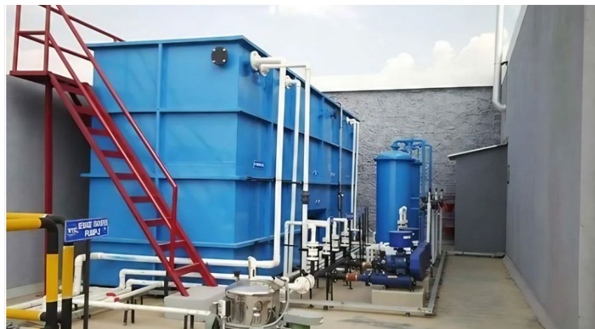
Image 1: 50KLD Pre-fabricated MBBR
