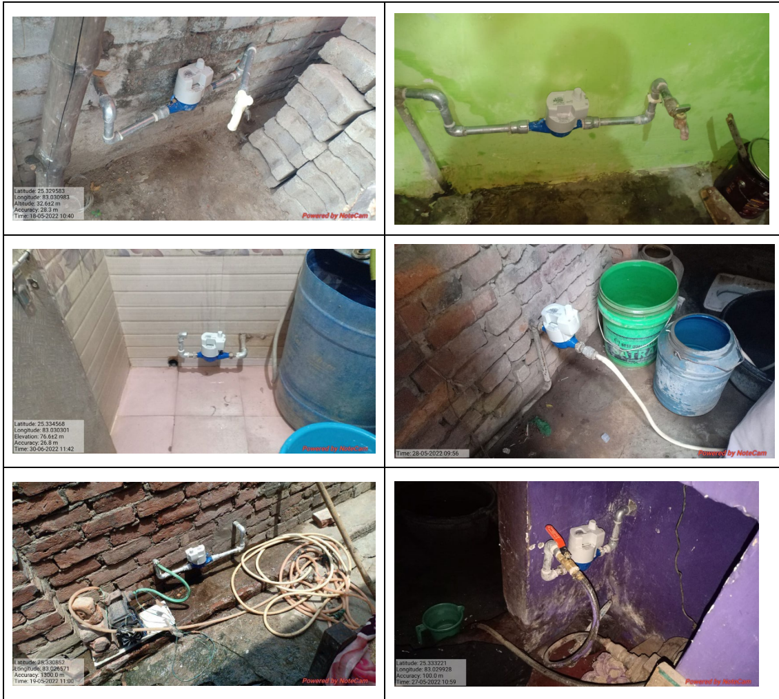
Figure 2-5. Photos of Customer meters installed in DMA.
