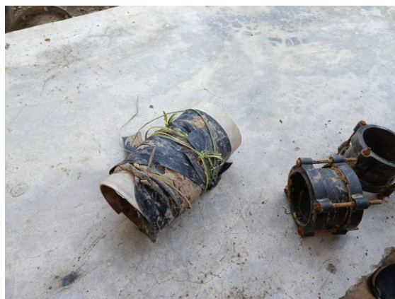
Figure 7-3. Inappropriate water stoppage method
