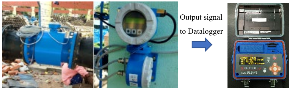
Figure 5-6. Portable Data Logger installed to the Electronic Magnetic Flowmeter at OHT
