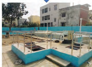
30KLD PSTU in Kanchanpur (Septage: 2KLD)
