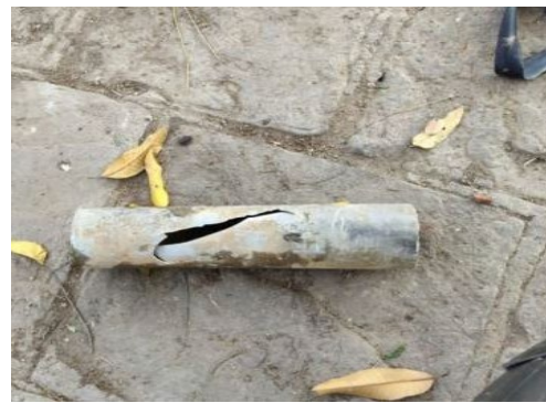
Figure 8-3. Damaged existing pipe
