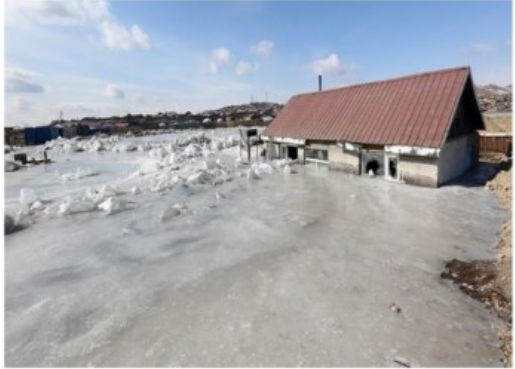
Figure 3.4.2 House damaged by Frozen Groundwater
