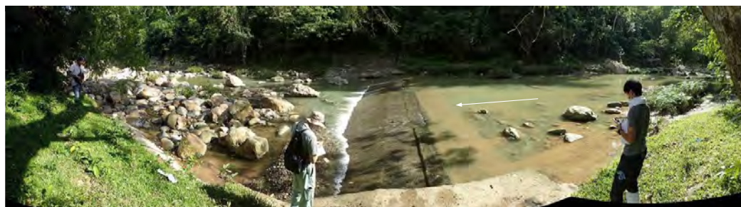
Site Inspection to Teruvian Weir in Kotkot River D/s of Kotkot Dam Site Dec. 09, 2022
